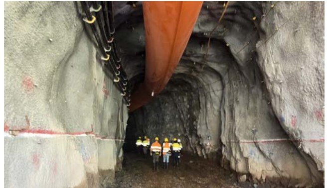
Figure 13: Very well laid out infrastructure. Nice an neat.
