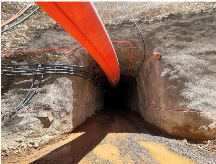
Figure 3: United North portal
